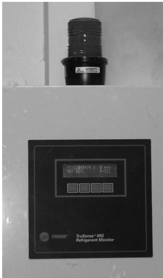
FIGURE 14.5 Alarm unit that detects leaks in poisonous gas.
