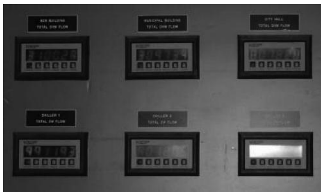
FIGURE 4.22 Display panel for a set of HVAC chiller units.
