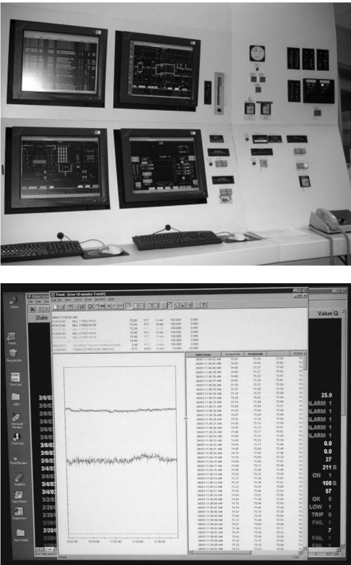
FIGURE 11.7 (Top) Four of six graphic user interface screens controlling a power plant with a few ancillary controls and displays, 2002 vintage. (Bottom) Screen 5 allows for clicking and expansion into a historical display.
